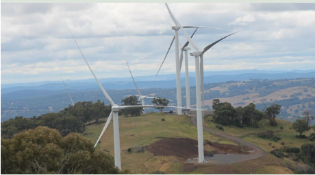
White Rock Wind Farm NSW
