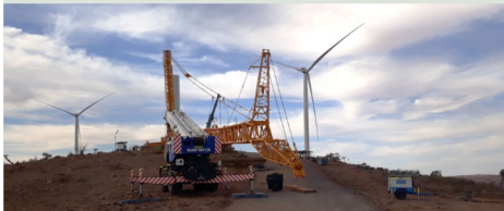
Silverton NSW – 200MW Stage 1 In operation (AGL Energy /PARF)
