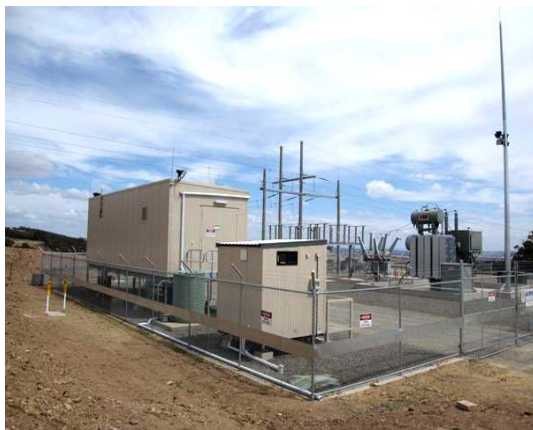
Plate 7 – Typical wind farm collector substation
