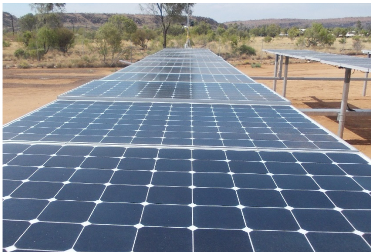
Photo 1. Example of a typical solar array
