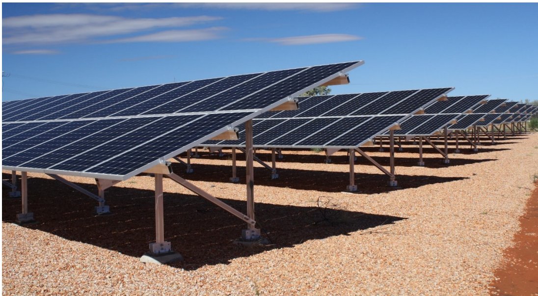
Photo 2. Example of a typical fixed tilt system
