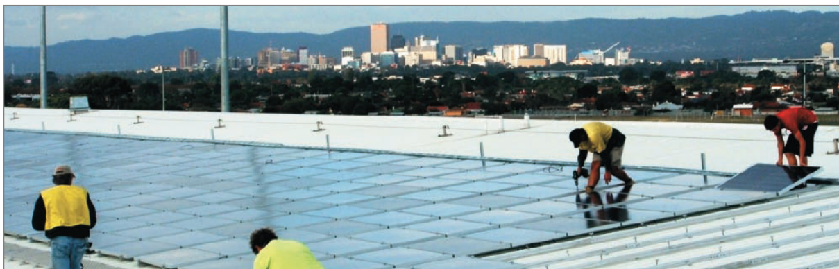
Figure 18 – Solar panels being laid on roof of Terminal 1, Adelaide Airport, 2008 Source: Solar Choice, www.solarchoice.net.au/blog/solar-panels-near-airports-glare-issue , 2013
