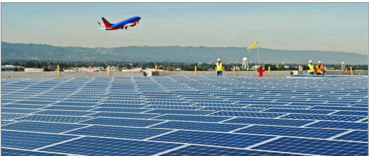
Figure 21 – Solar panels on roof of Rental Car Center, San Jose International Airport, 2010 Source: Solar Choice, www.solarchoice.net.au/blog/solar-panels-near-airports-glare-issue , 2013
