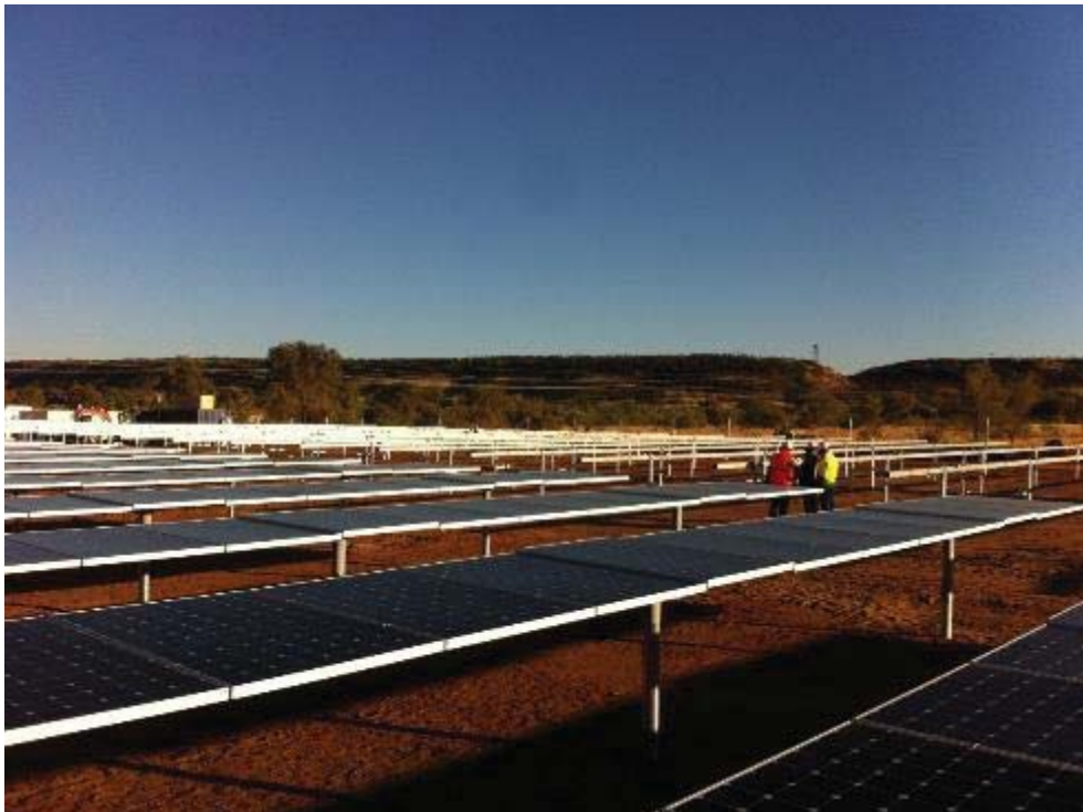
Figure 3-10 Example of solar array
