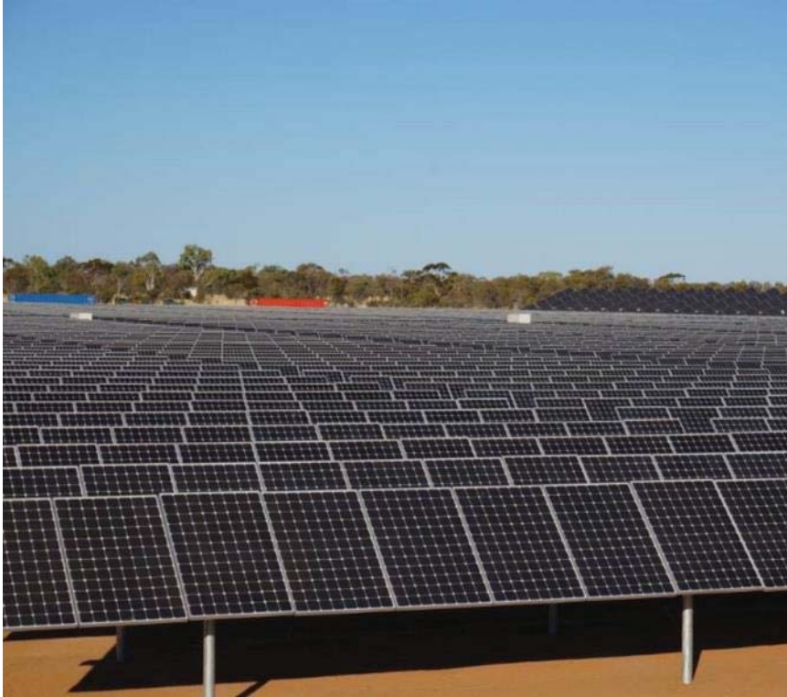
d) The operational solar array
