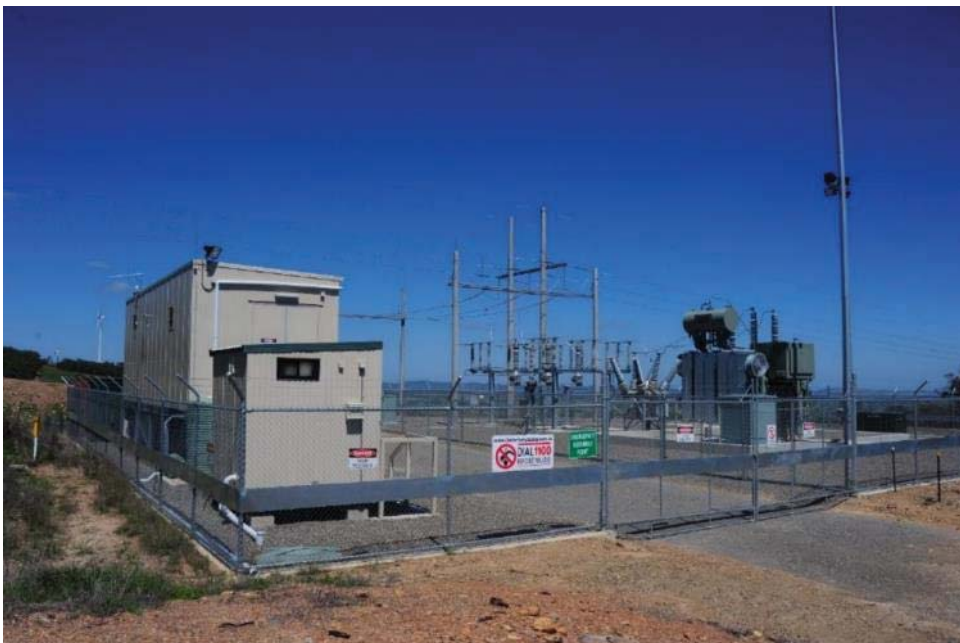
g) Example onsite substation
