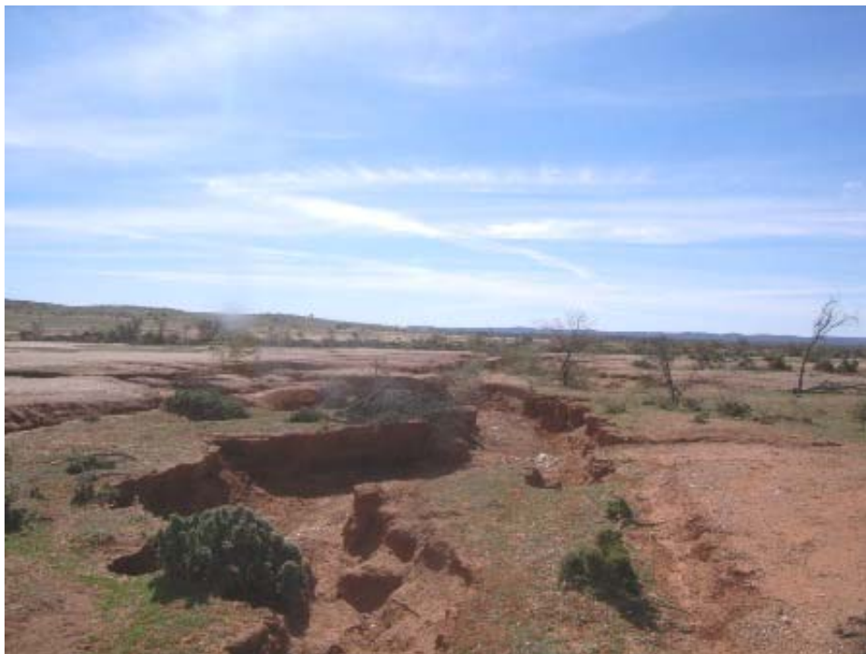
Plate 4. Looking north from the same location as Plate 3 showing the extensive, erosion of the alluvial landform 30 m below the knick point.
