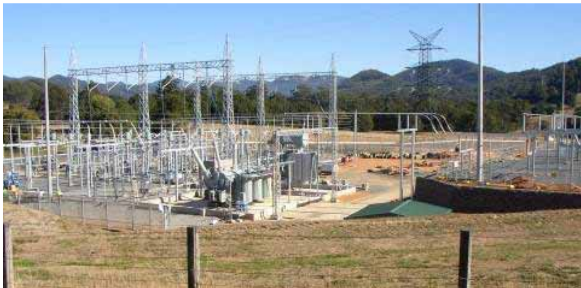
Figure 3-12 Coffs Harbour 330/132kV substation (courtesy TransGrid)
