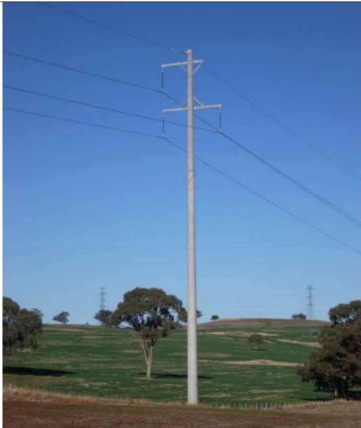
Plate 1.1 Existing Single circuit 132kV transmission line near the existing 330kV transmission line on skyline
