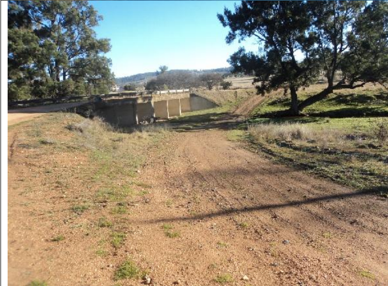
Plate 7.10 – Spring Mountain Road bridge over Swan Brook showing low level bridge bypass on eastern side of bridge.
