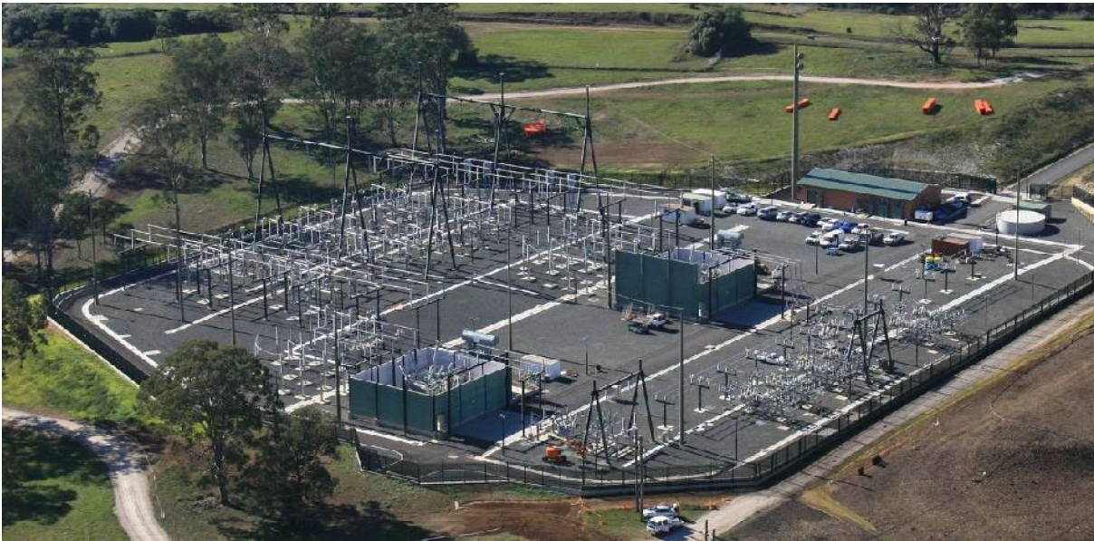
Plate 3-2 – Example 330kV substation (Macarthur) constructed in Sydney by TransGrid in 2009
