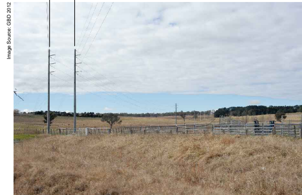
Double circuit 132kV transmission line (angle pole structure) at road crossing
