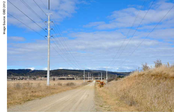
Double circuit 132kV transmission line (supporting structure) along road
