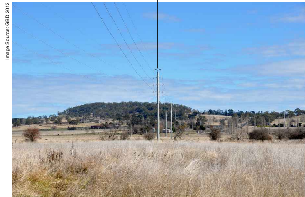
132kV double circuit line crossing rural agricultural land
