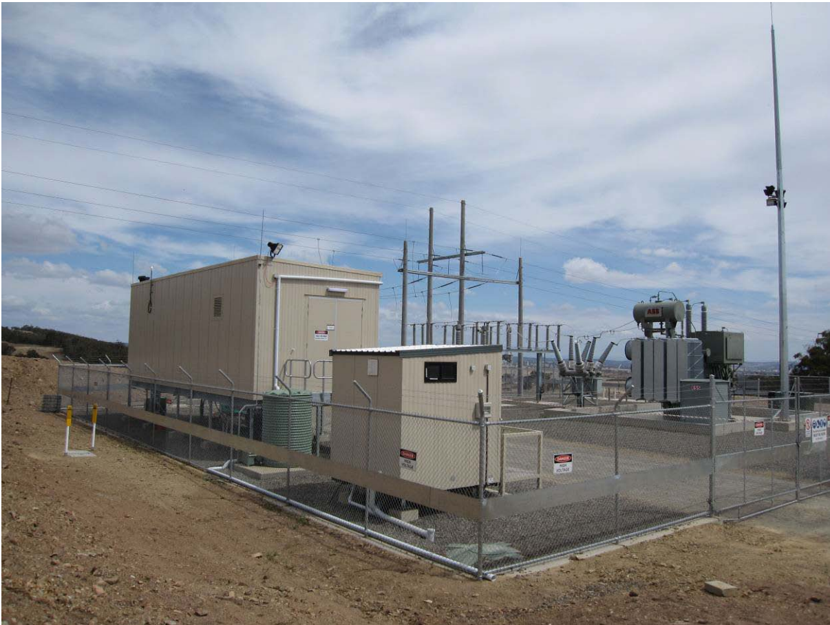
Figure 3-7 Cullerin Range Wind Farm 132/33kV site substation
