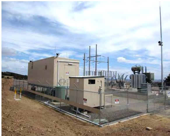
Plate 7 – Typical wind farm substation
