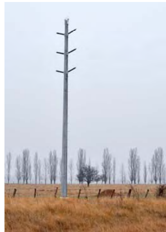
Plate 8 – Typical 132kV supporting structure
