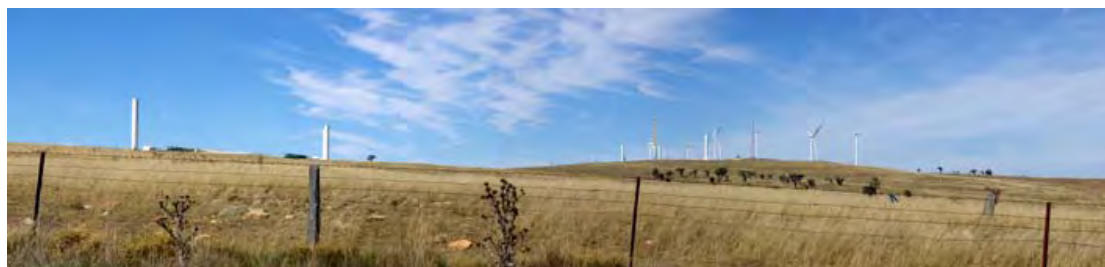
Plate 10 - Illustrating general construction activities at the Capital Hill wind farm site, including views toward cranes, partial construction of towers and laydown areas.
