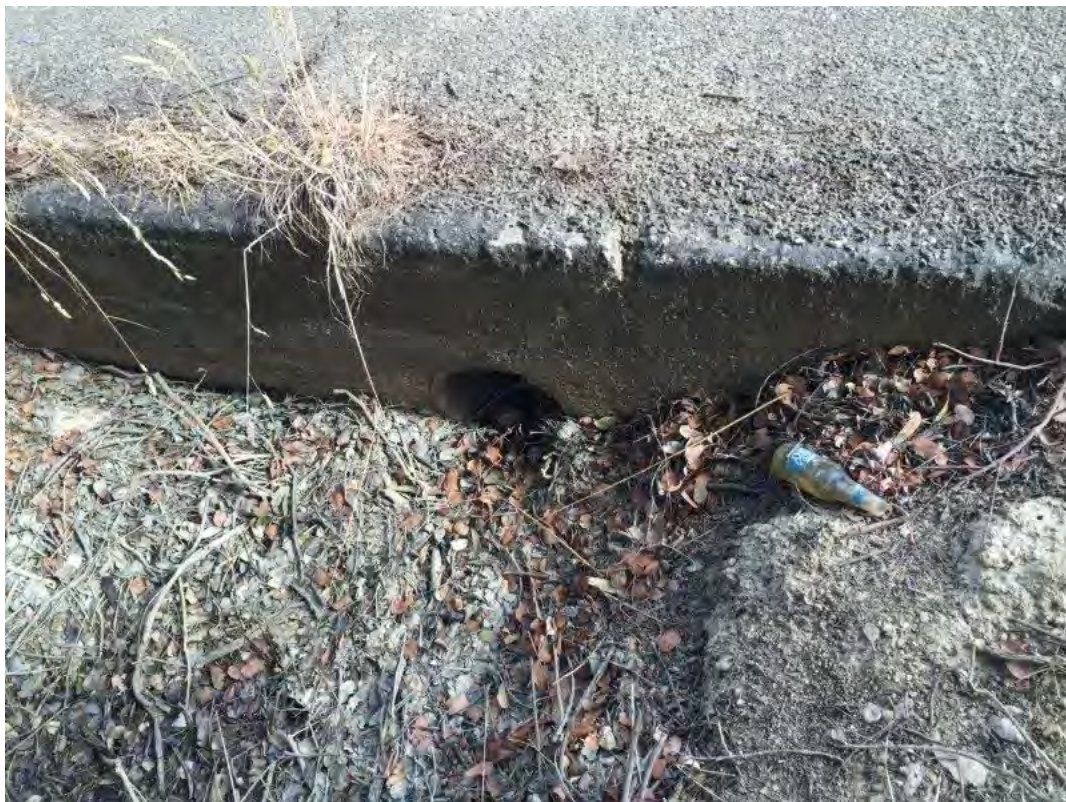
S002 – Causeway Low Flow Pipe
