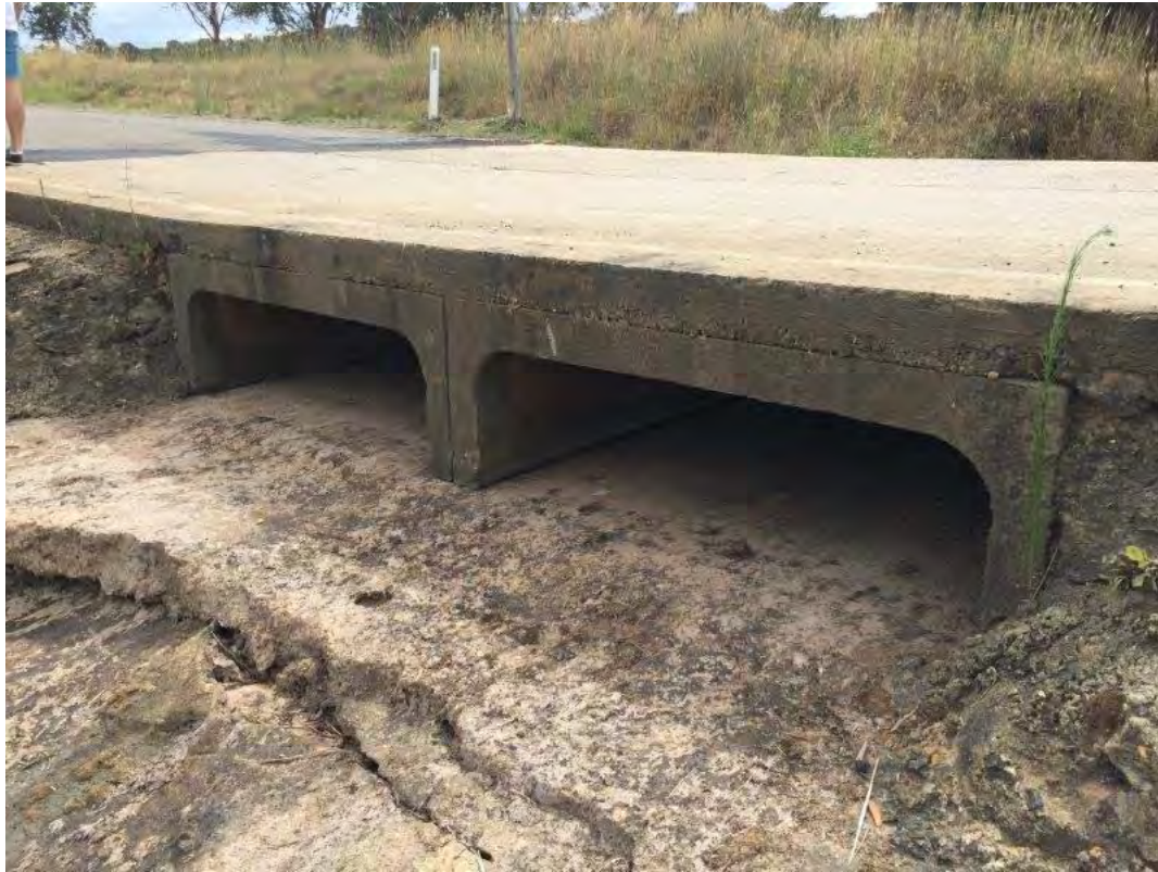
S007 – Low Flow Culverts
