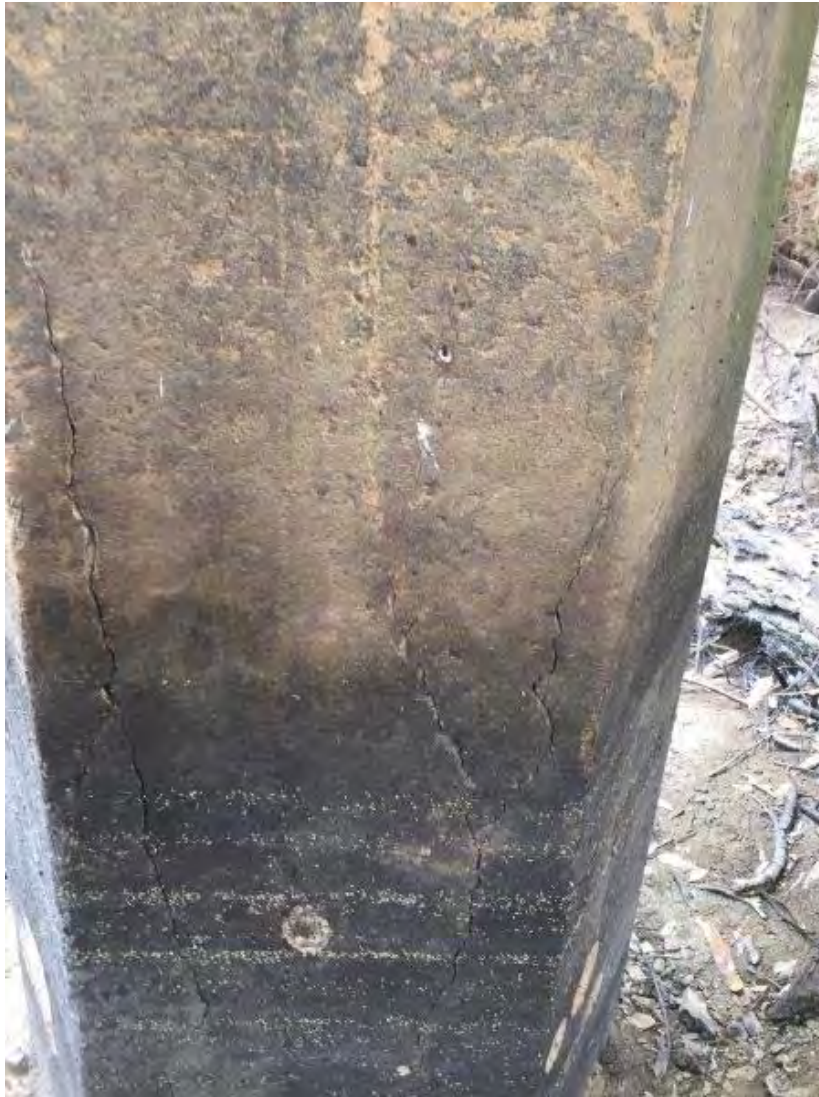
S010 – Bridge Column, Vertical Cracking, Typical each face and both Columns
