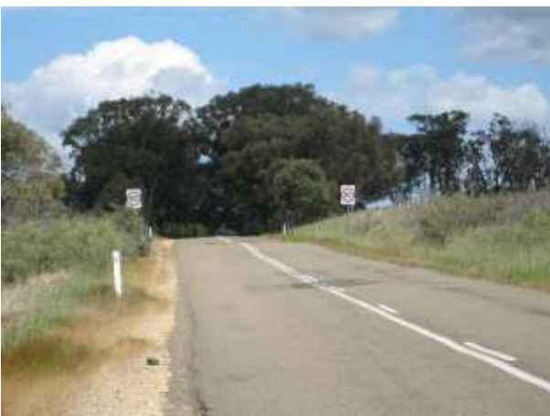
PLATE 17 Burrinjuck Road failing pavement
