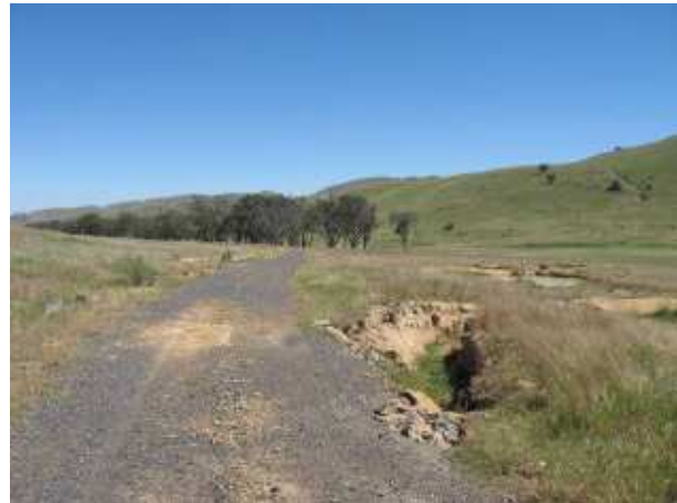
PLATE 52 Whitefields Road erosion at 3.33km.
