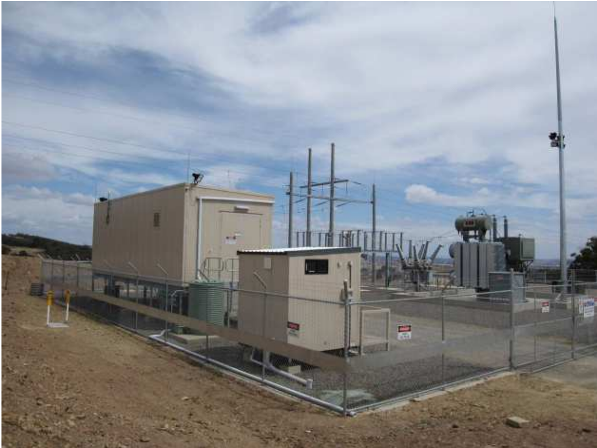
Figure 3-13: Cullerin Range Wind Farm 132/33kV substation
