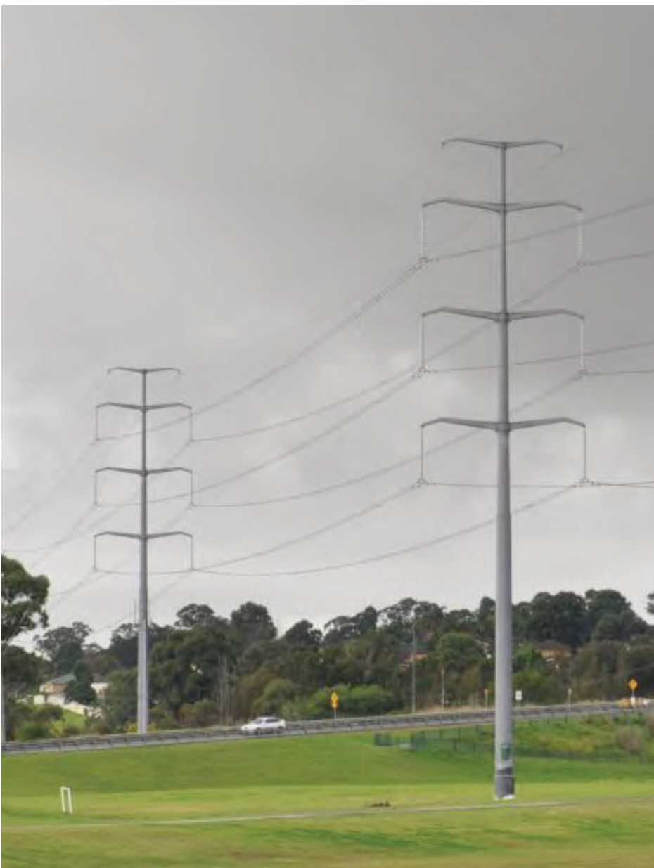
Figure 2-5 Example of a double circuit 330 kV overhead powerline mounted on a single pole type structure
