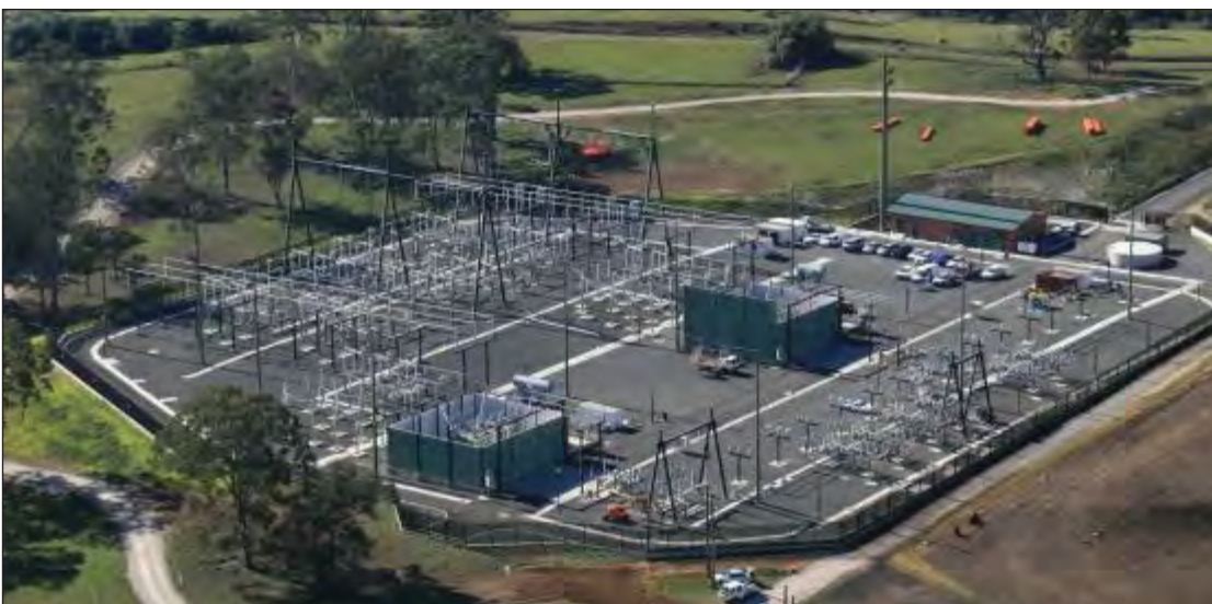
Figure 2-3 TransGrid's 330 kV Macarthur Substation in southwestern Sydney
