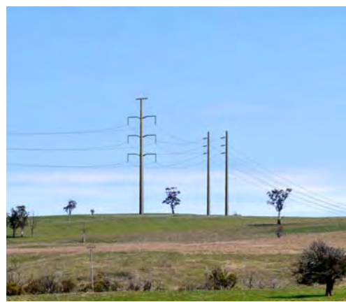
Plate 8 – Typical illustration of a 330 kV supporting structure and angle poles
