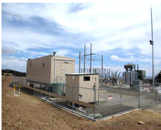
Plate 7 – Typical wind farm collector substation
