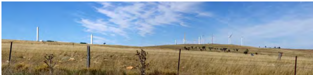
Plate 12 - Illustrating general construction activities at the Capital wind farm site, including views toward cranes, partial construction of towers and laydown areas.
