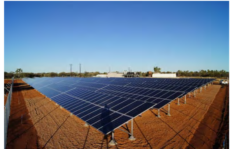
TKLN Solar Project Northern Territory
