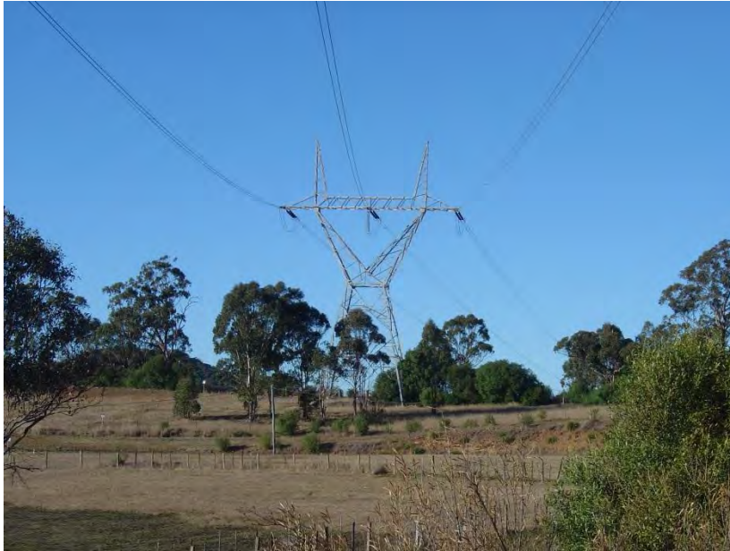
Example of 330kV transmission line tower structure
