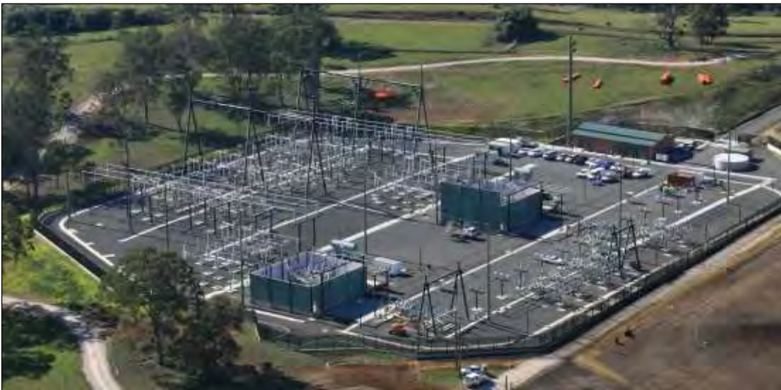
Figure 3-14 TransGrid's 330 kV Macarthur Substation in western Sydney
