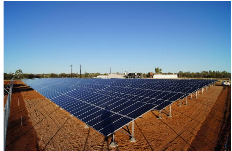
TKLN Solar Project Northern Territory
