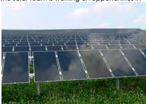
Photovoltaic Modules (PV)
