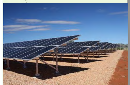
TKLN Solar Power plant, Kalkarindji, NT
