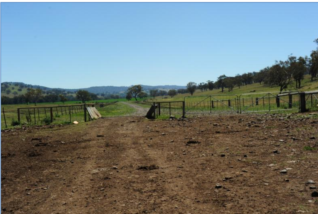
Figure 4-7 Unsealed section of Rotherwood Road
