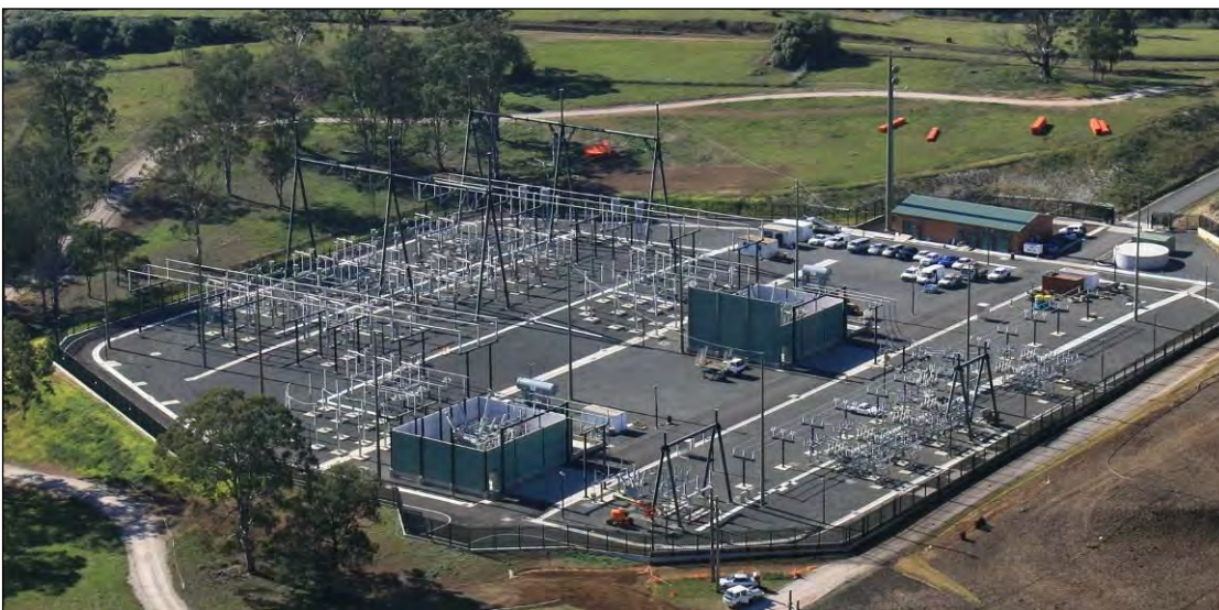
Figure 3-10 TransGrid's 330 kV Macarthur Substation in western Sydney
