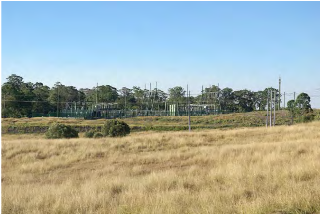
Plate 14 –Typical illustration of a 330 kV substation
