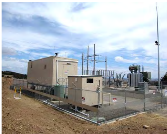
Plate 11 – Typical wind farm collector substation
