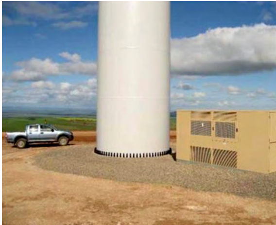
Plate 13 – Typical of a generator transformer
