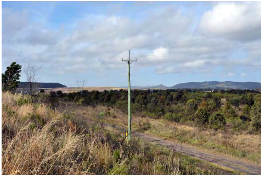
Plate 17 Illustrating typical electrical infrastructure at the Ulan colliery site.
