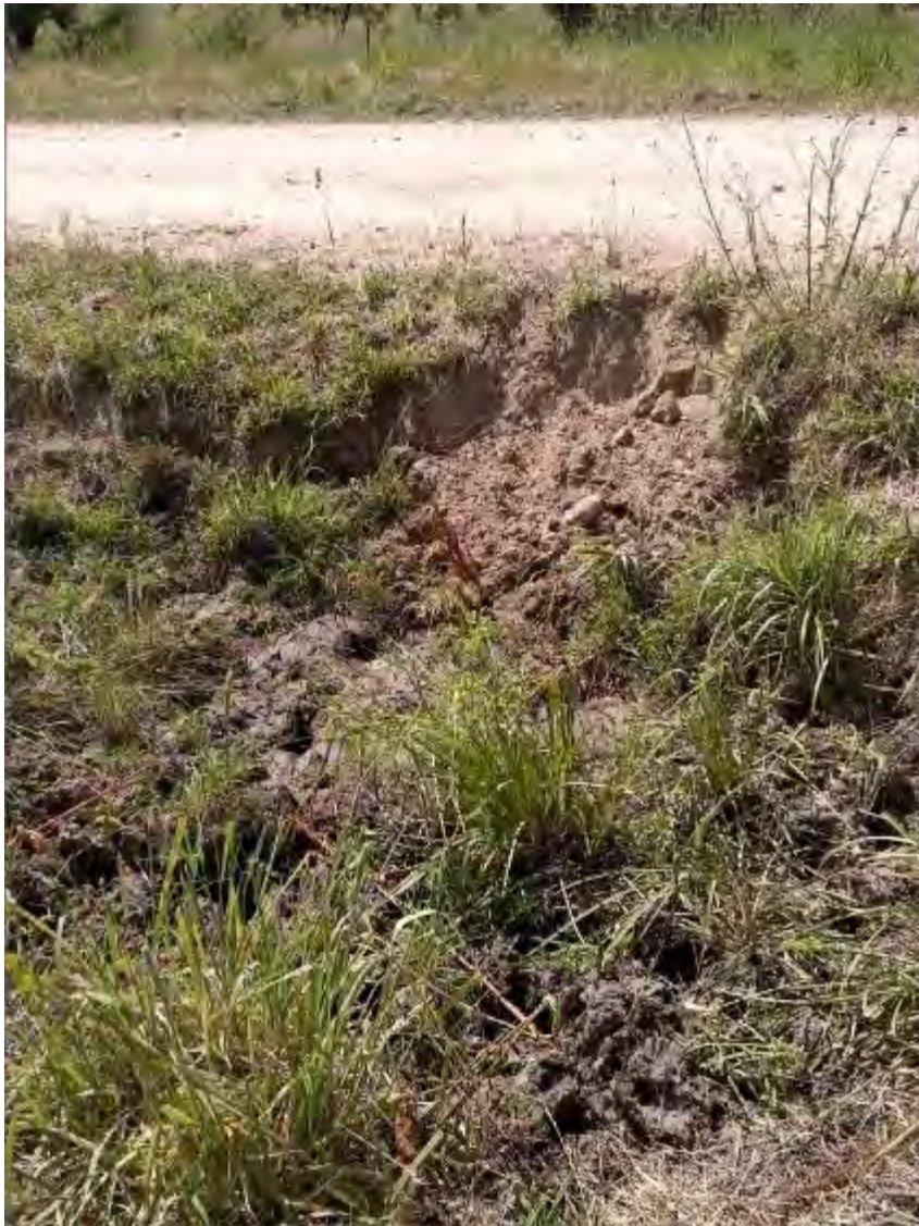
S151 – Blocked Pipe Culvert
