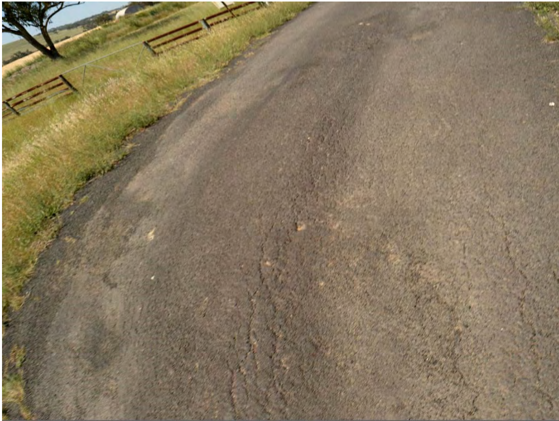
S146 – Road showing Cracking/Ravelling
