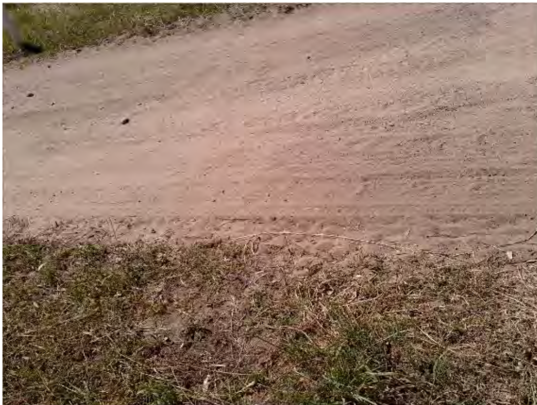
S154 – View of Causeway, Water damage shown on close side
