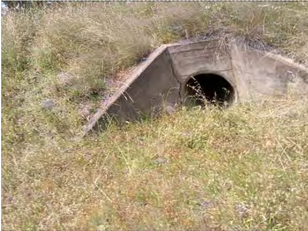
S186 - 750mm Pipe Culvert with cracked headwall
