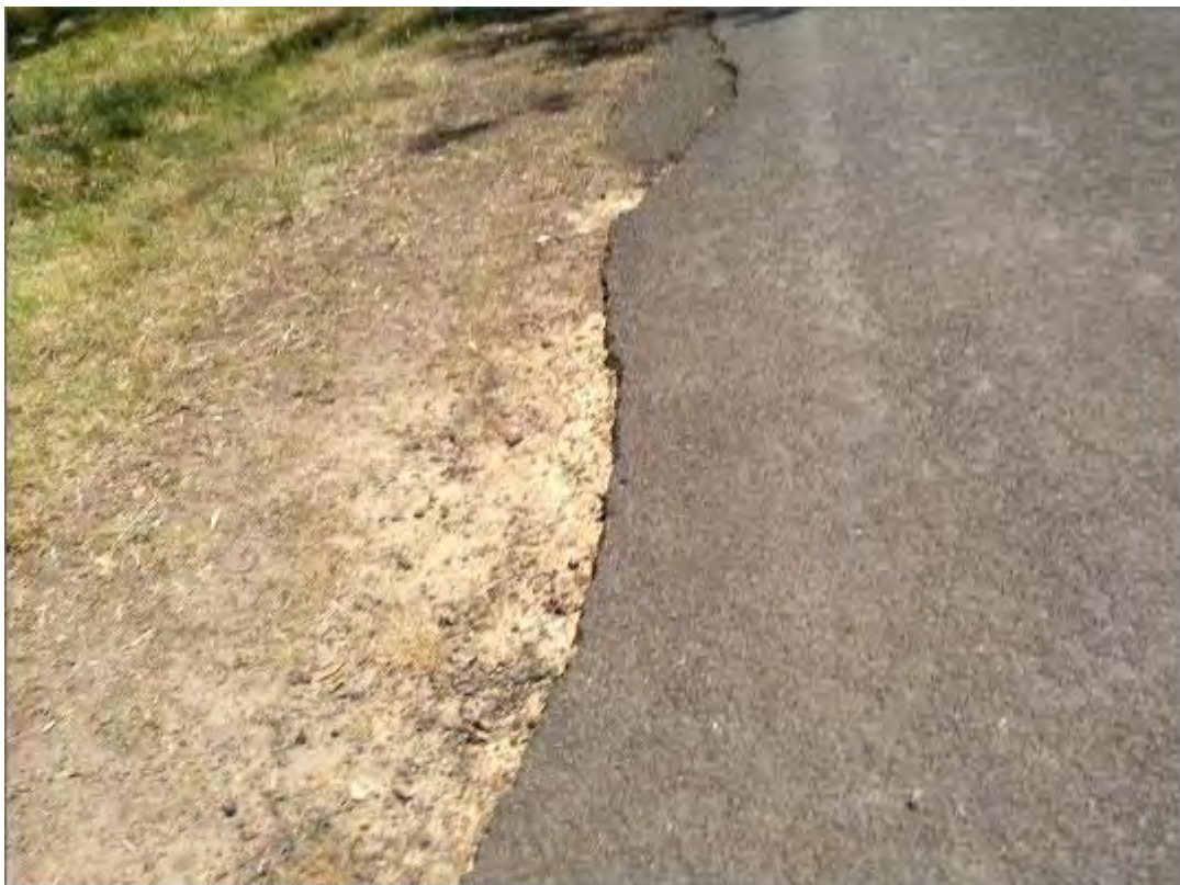
S145a – Road showing Edge Break
