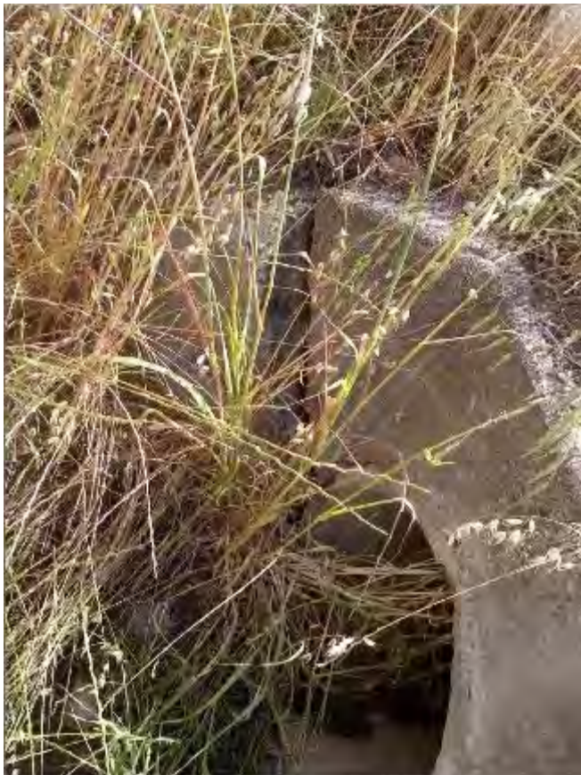
S099 – Broken Headwall
