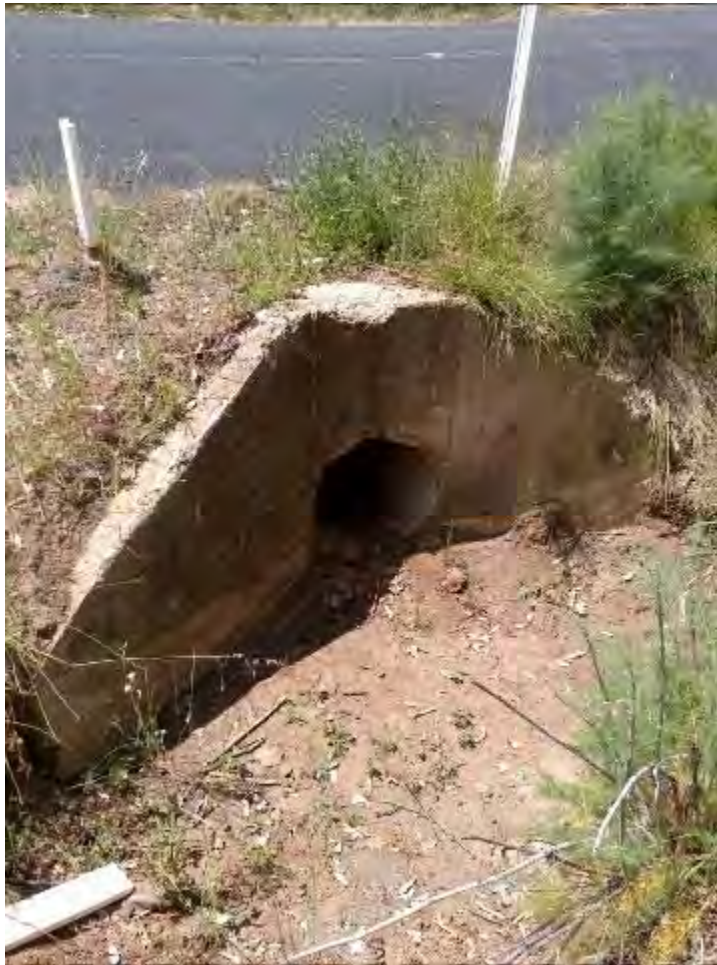
S109 – 600mm Blocked Pipe Culvert
