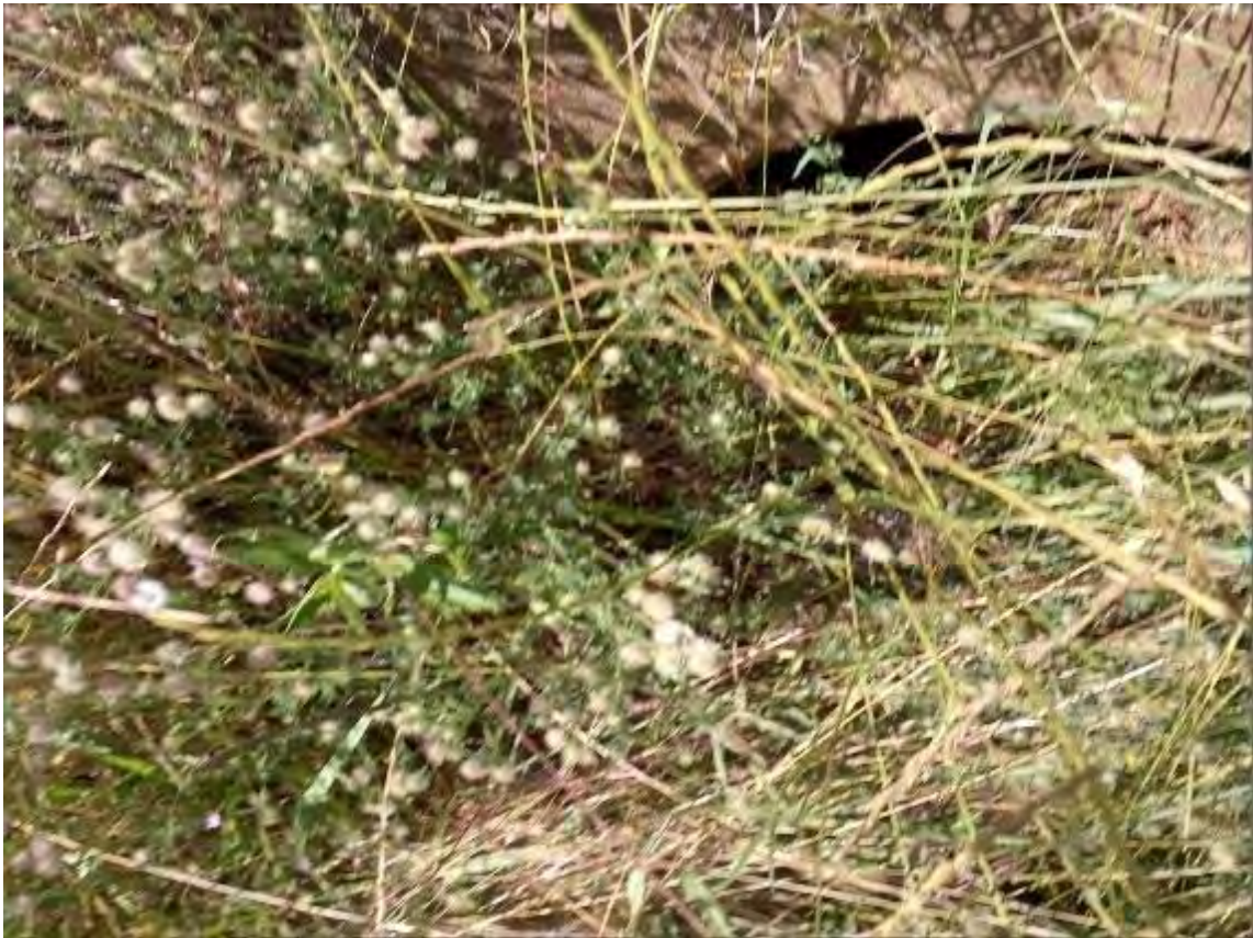
S125 –450mm blocked pipe culvert
