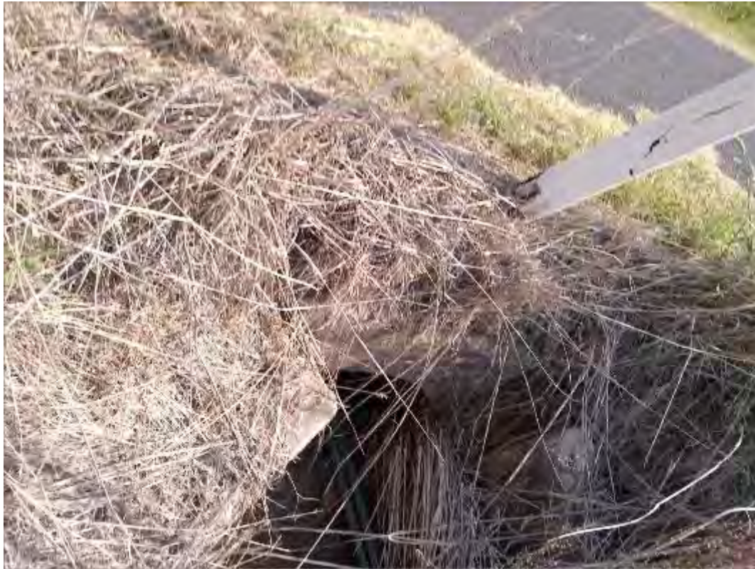
S076 - 450mm Pipe Culvert with broken headwall
