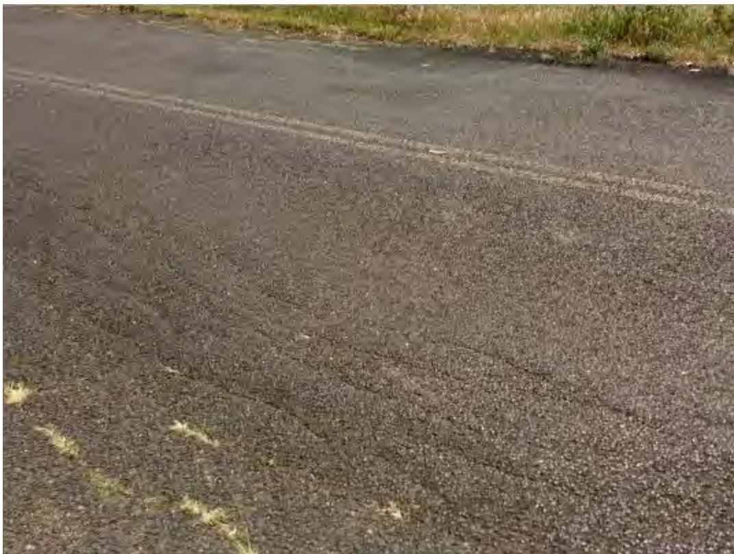
S119 – Road showing signs of wear
