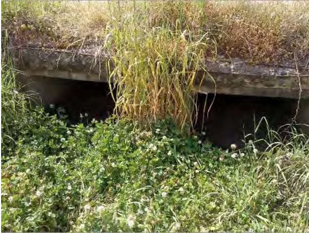
S089 – 2 of 750mm by 1200mm reinforced concrete box culvert
