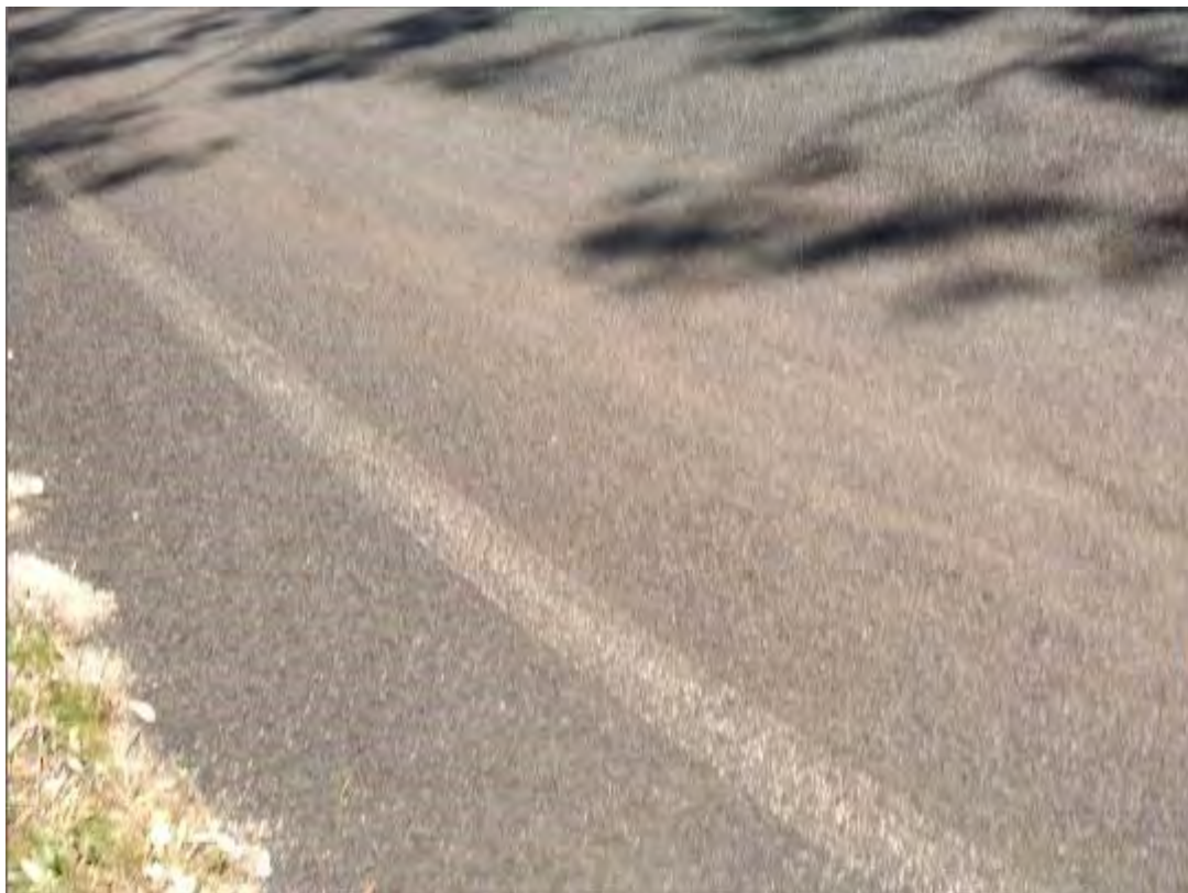
S112 – View of Causeway showing signs of rutting
