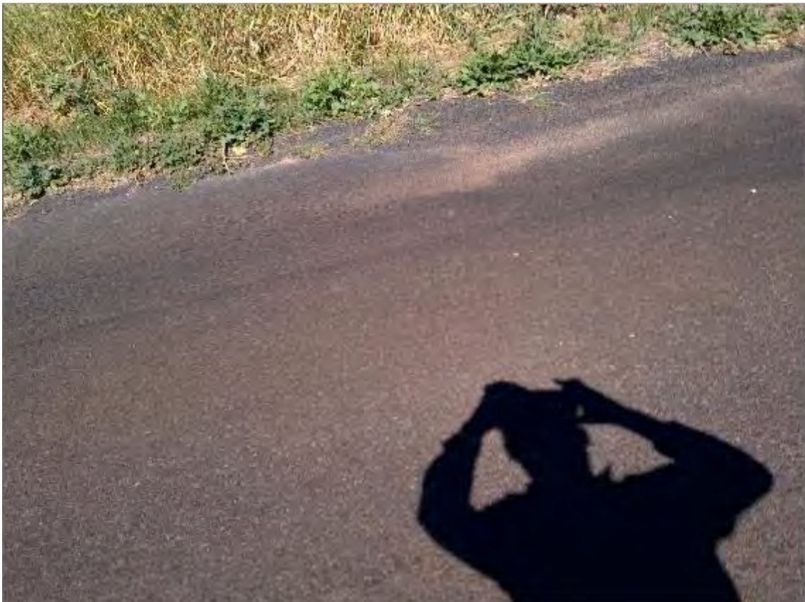
S127 – Pothole on Road Caused by Rutting
