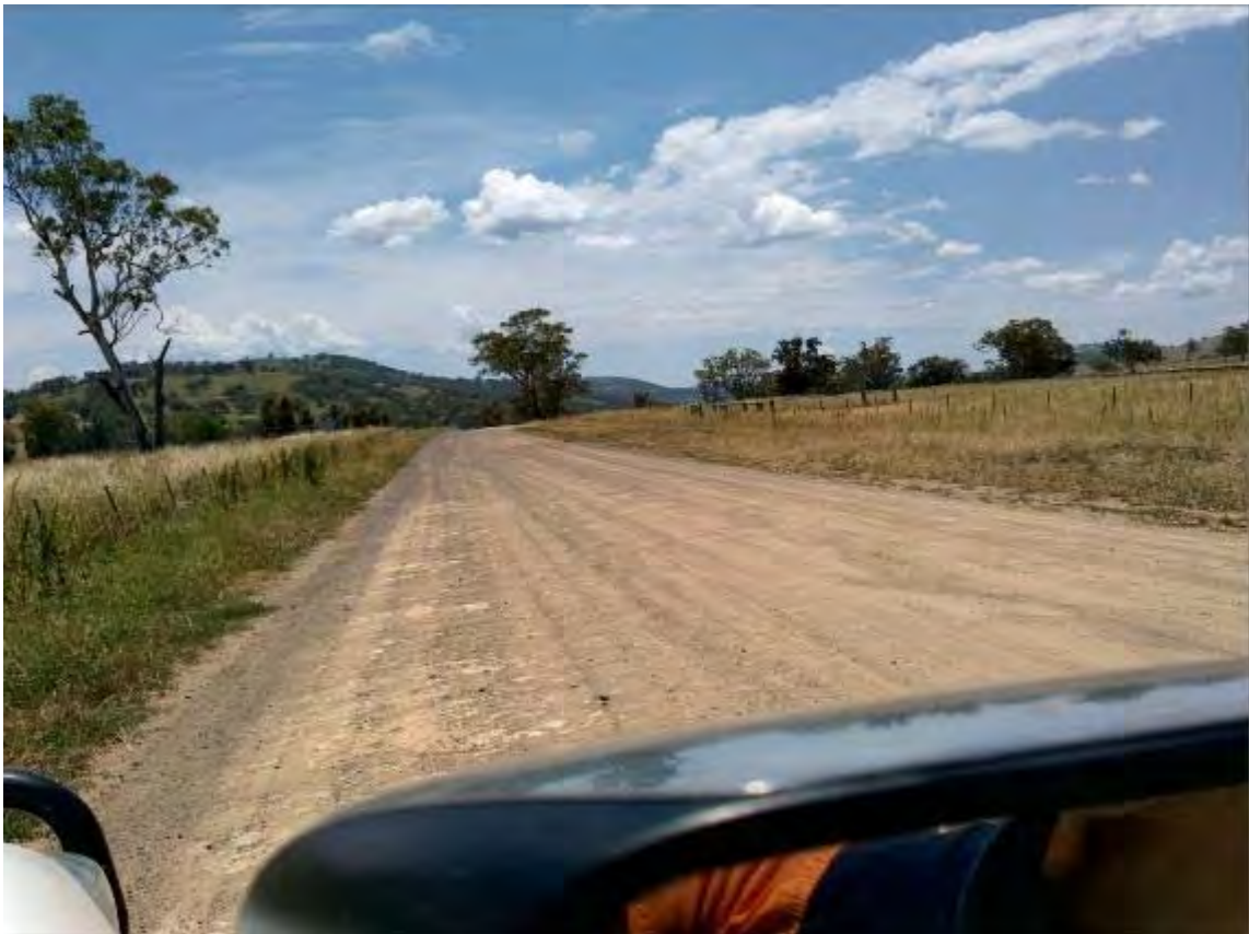
S213 – Water Damage on Road
