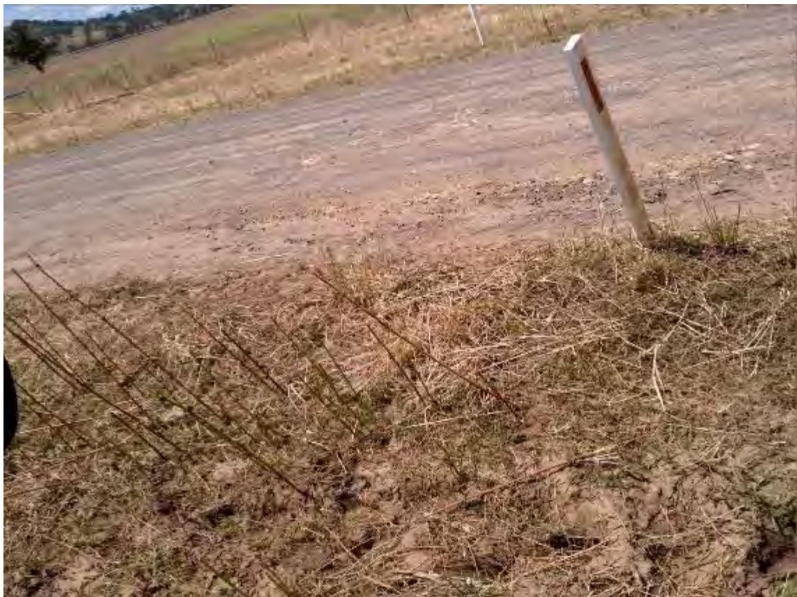
S212 – Blocked Culvert at bottom of image
