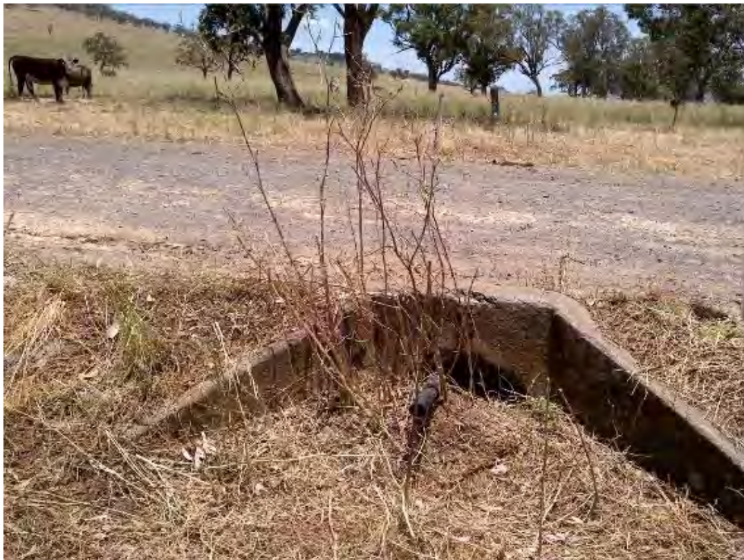
S216 – Blocked 450mm Pipe Culvert
