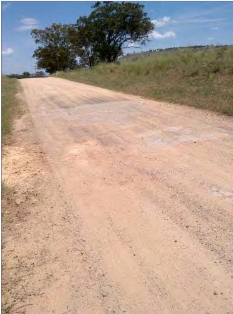
S231 – Causeway with damages
