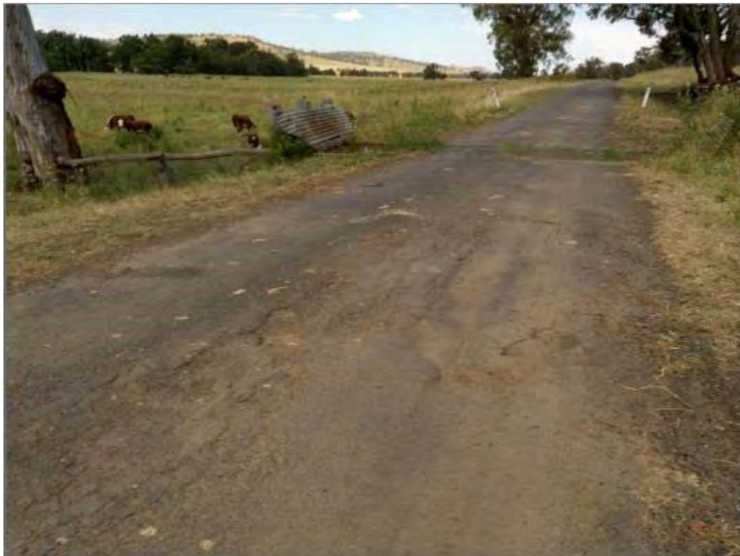
S201 – View to North, Location of Culvert Shown at Top Right of Image
