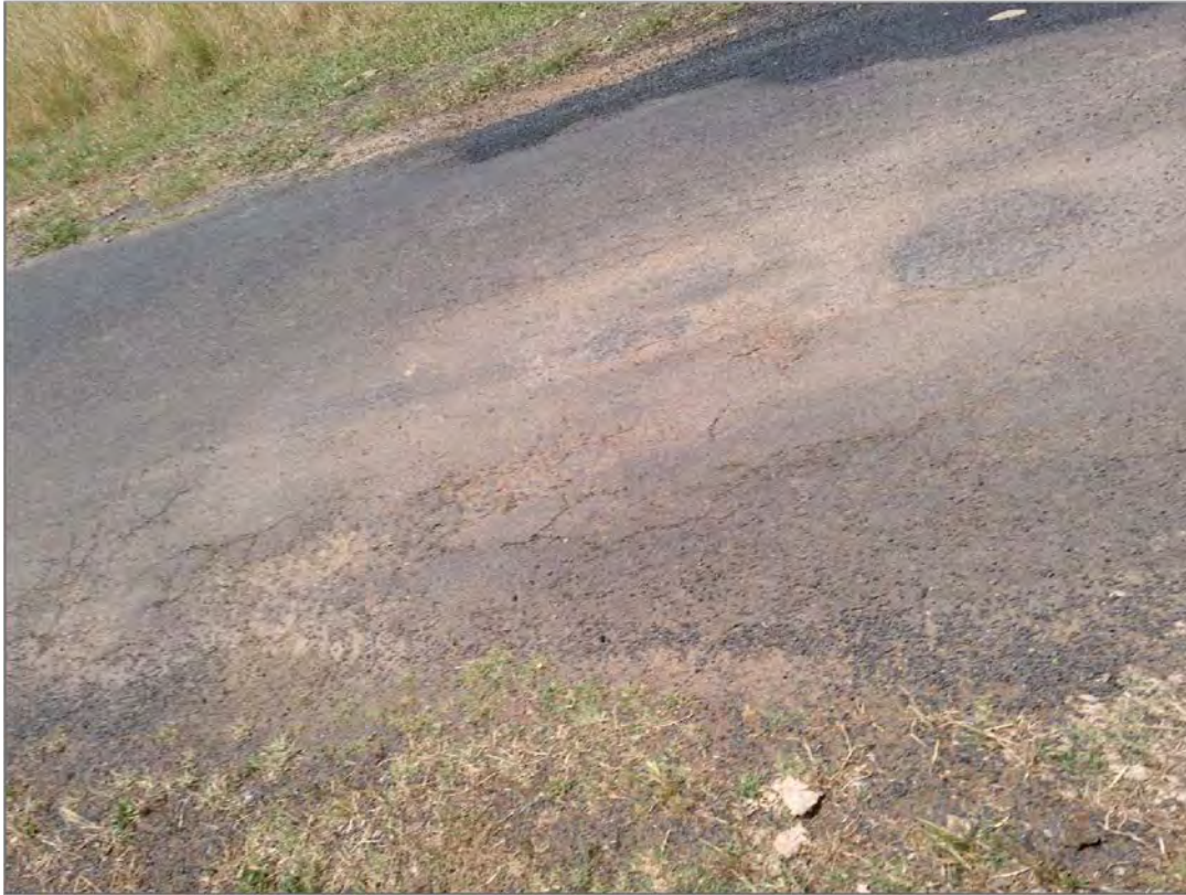
S203 – Damage on Road due to Floodway
