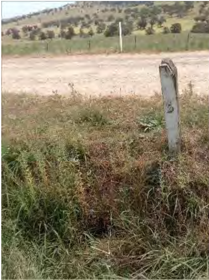
S242 – Overgrown Culvert
