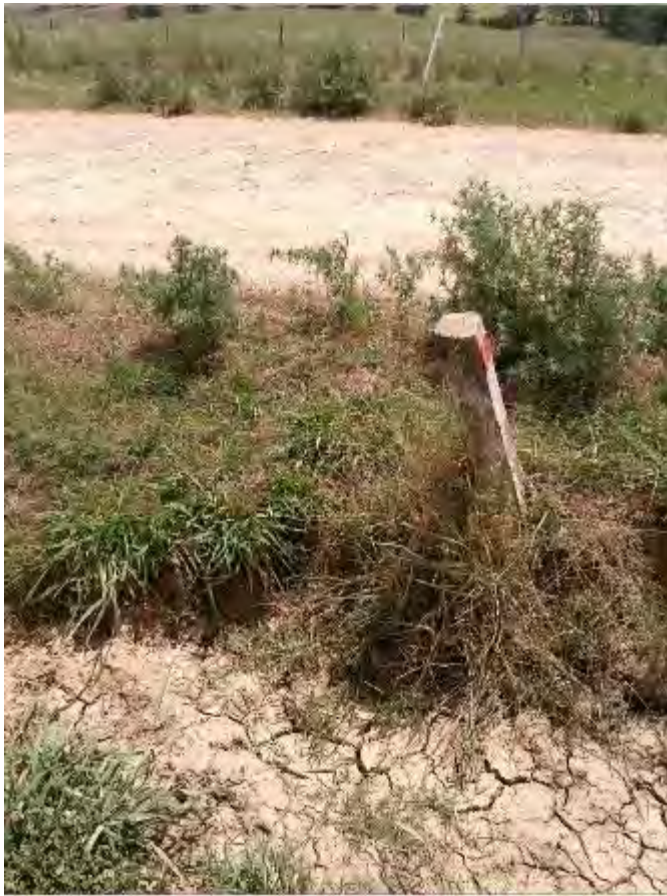
S243 – Blocked Pipe Culvert
