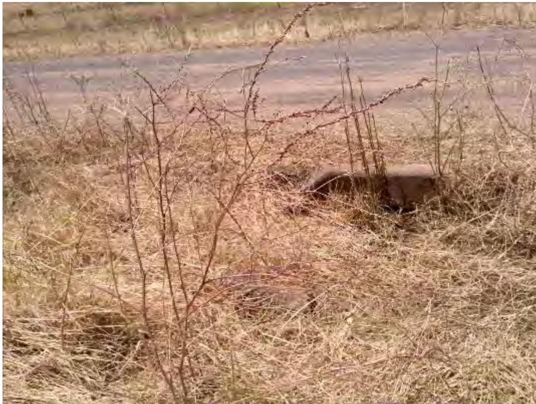
S209 –Blocked Pipe Culvert
