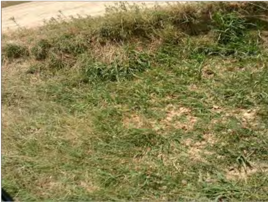
S246 – Blocked Pipe Culvert
