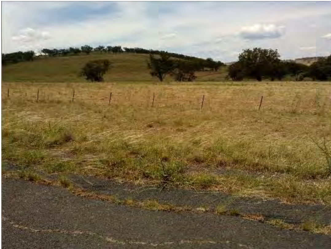
S223 – Road has signs of cracking and it being overgrown
