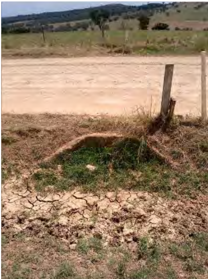
S245 – Blocked Pipe Culvert
