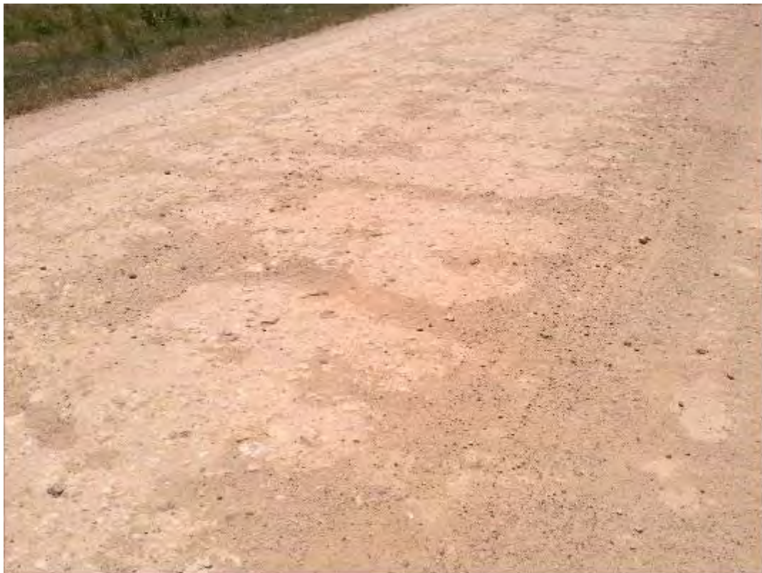
S232 – Road in poor condition
