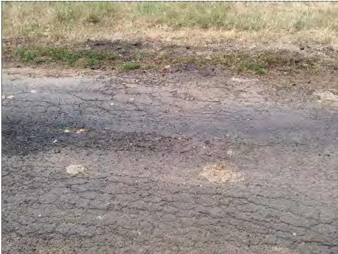
S201 – Road badly damaged at Location, Rutting and Extreme Cracking shown above, also signs of Stripping
