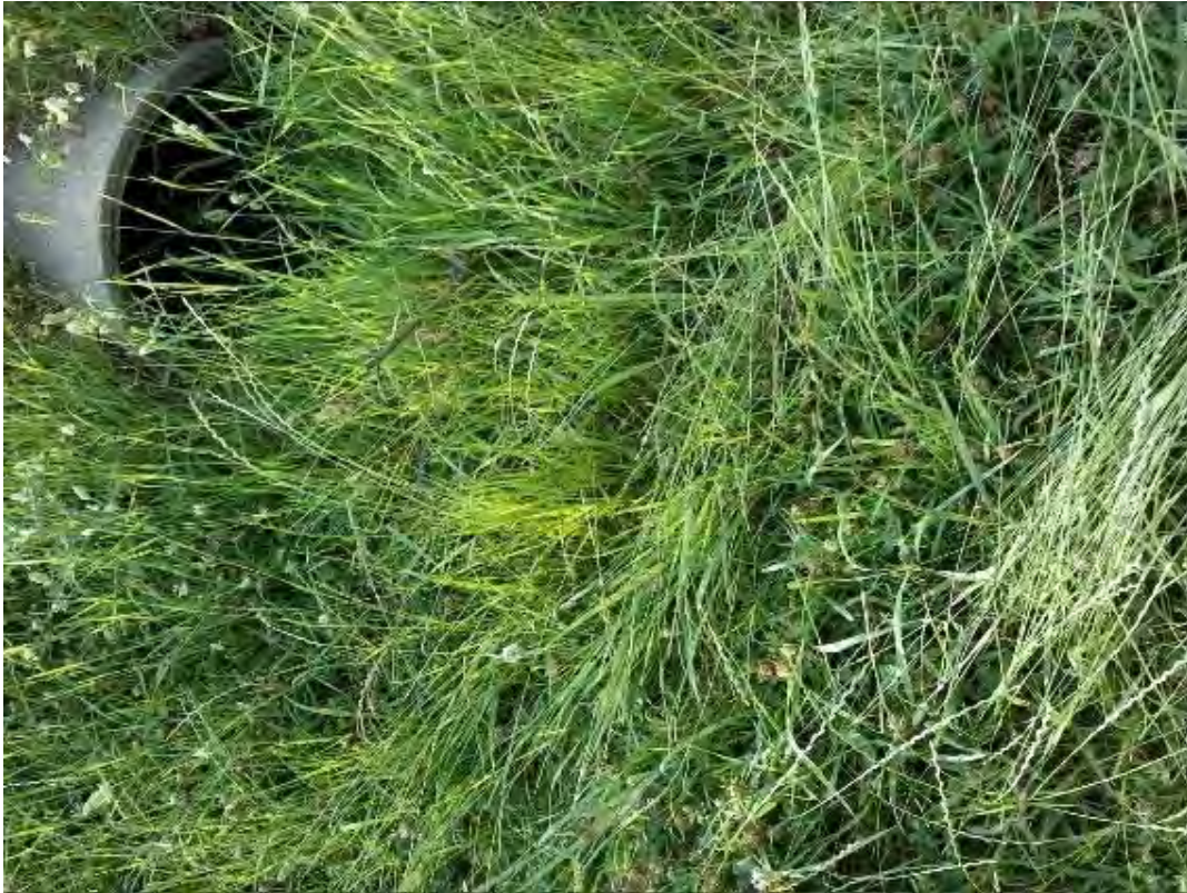
S059 – 600mm Pipe Culvert no headwall
