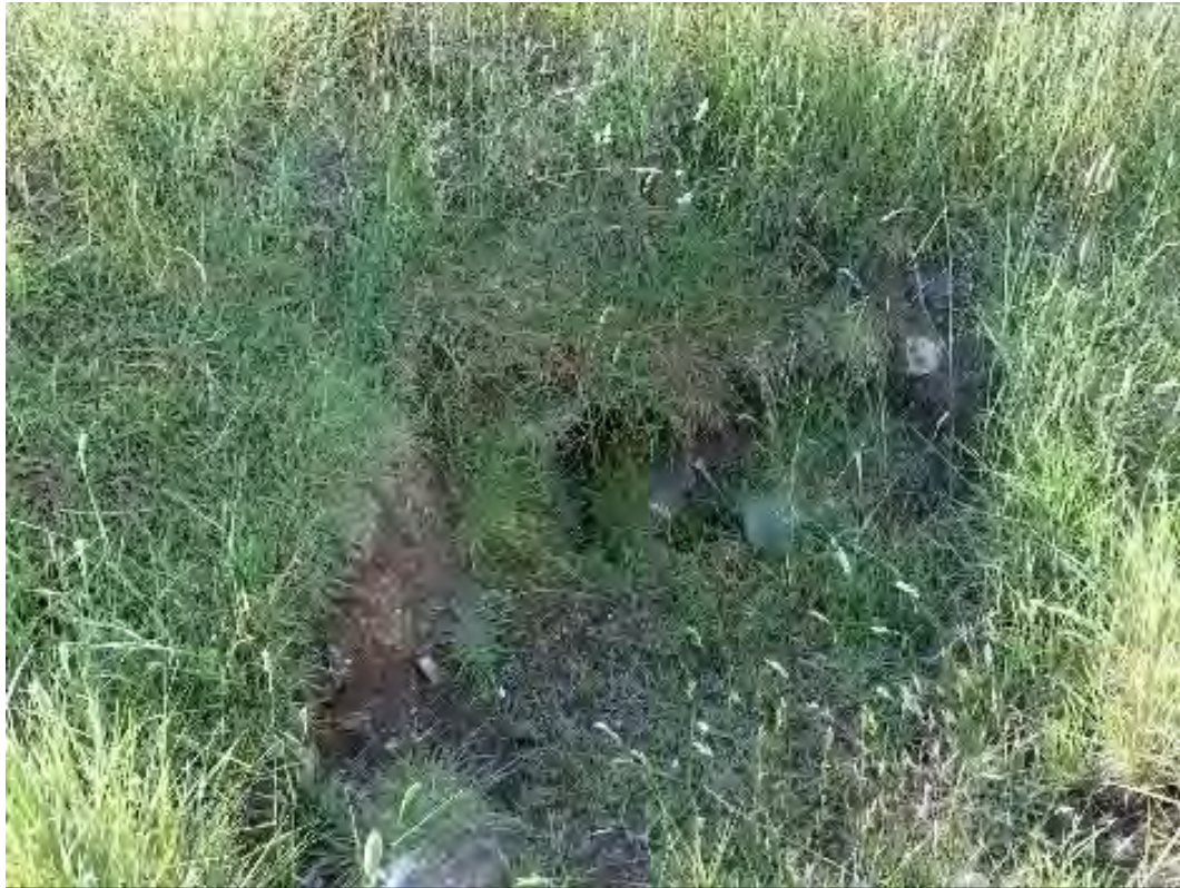
S056 – 375mm Pipe Culvert with no headwall
