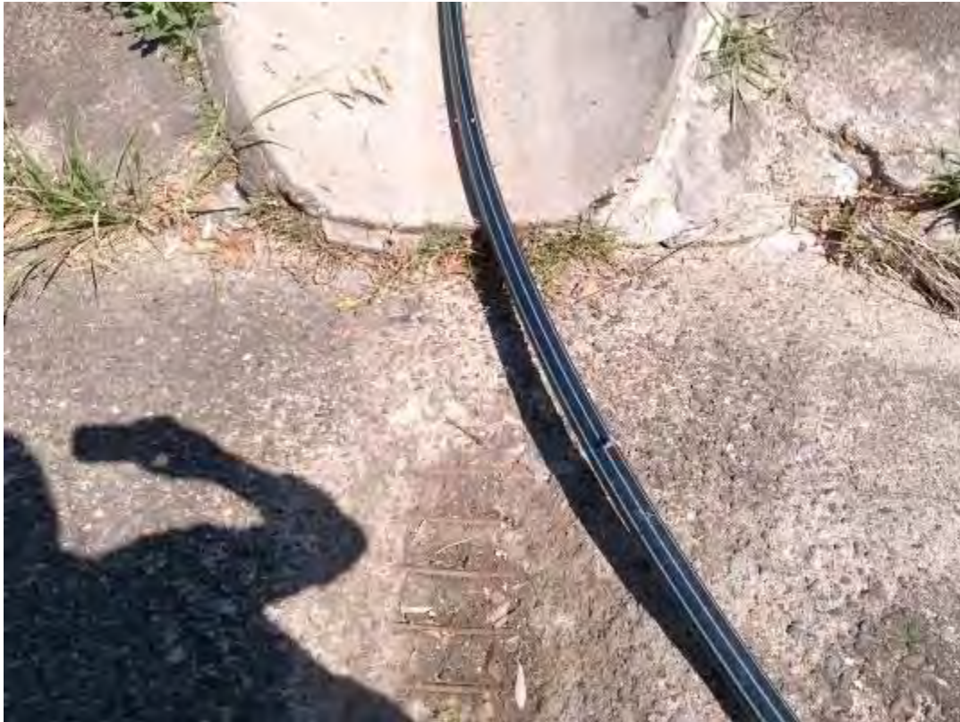
S037 – High flow water has eroded the concrete exposing the reinforcing Steel
