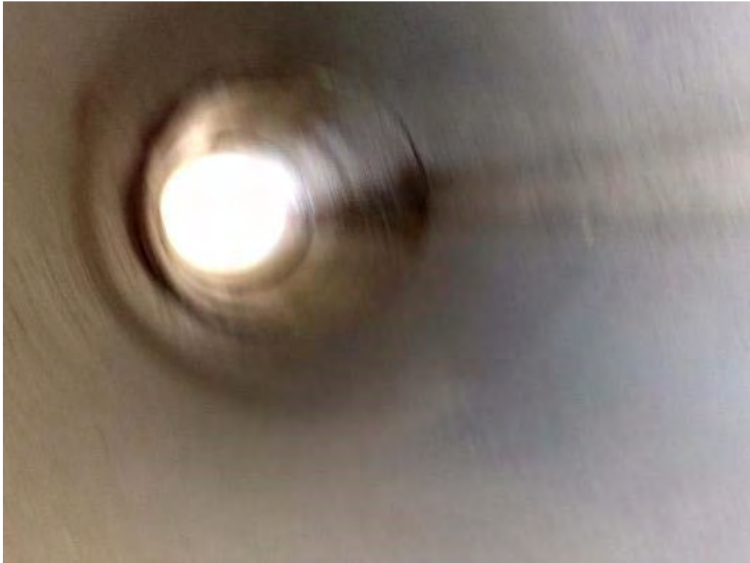
S007 – Internal View, Crack shown along circumference at Mid-Length
