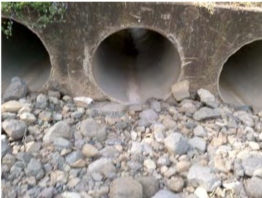
S007 - 3-1050 Pipe Culvert, Crack shown on bottom side of middle Culvert
