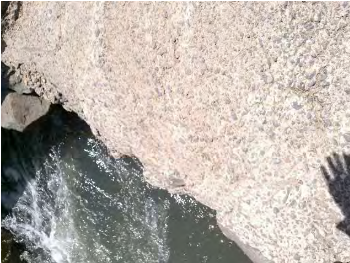
S025 – Edge of culvert is worn.
