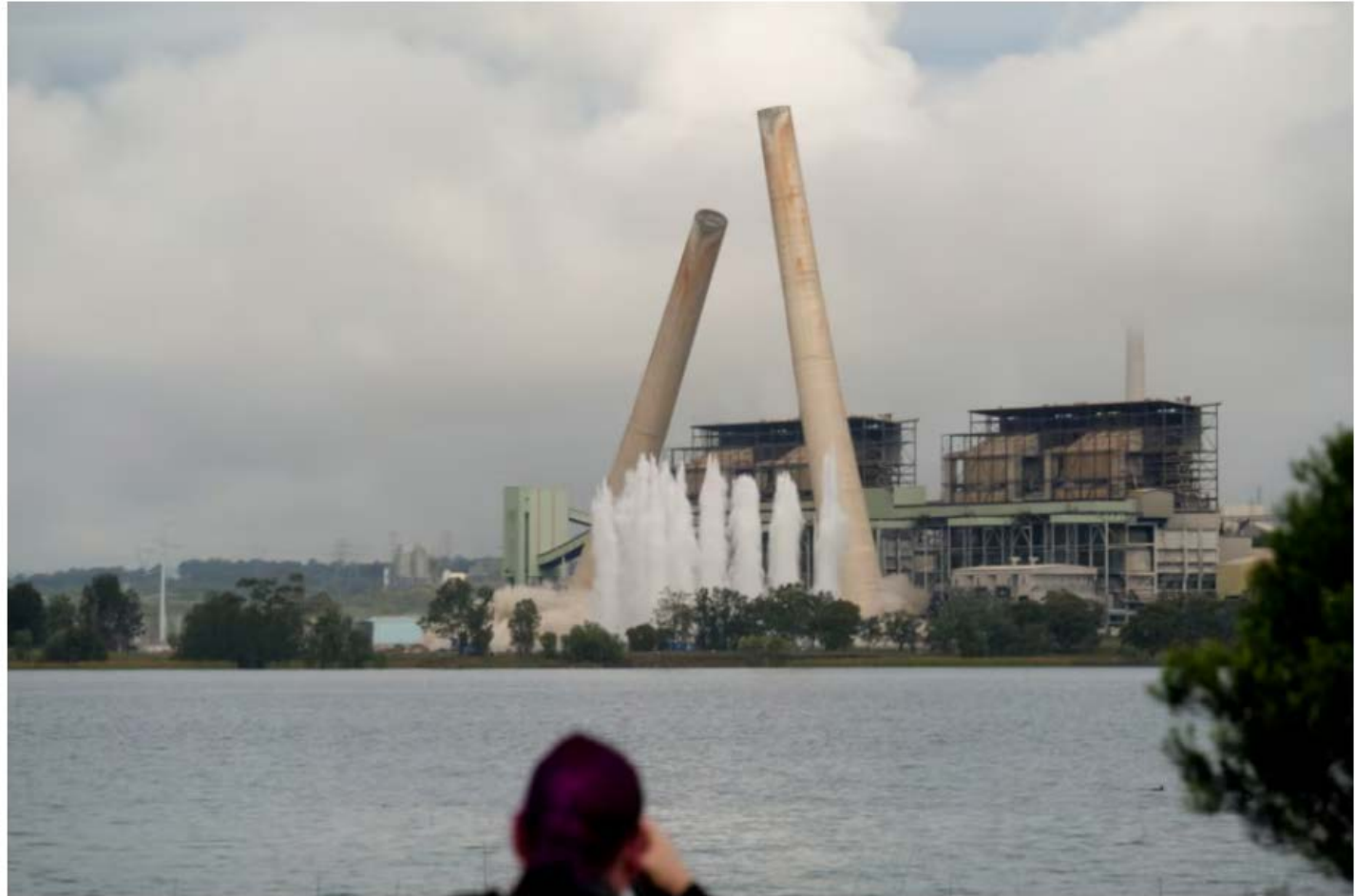
The moment the chimneys at the Liddell power station were demolished. (ABC Newcastle: Amelia Bernasconi)
