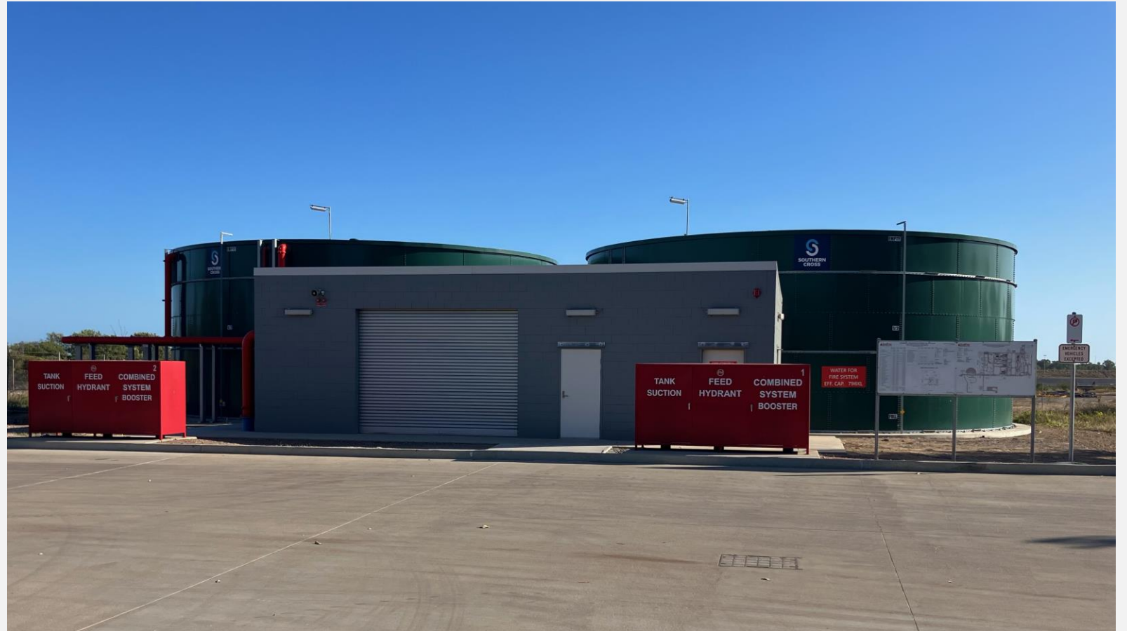
Pump Station (Sun Metals Corporation) – recently commissioned with 2 × 796KL water storage tanks for fire fighting and training purposes
