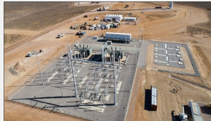
Collector substation – including 33/330kV power transformers
