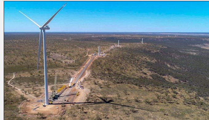
Hardstands - crane pad & equipment laydown area (blades, tower, nacelle etc.); 1.5 to 2 ha per turbine.
