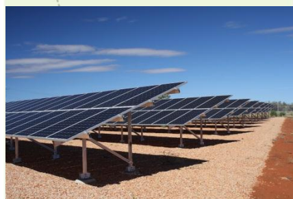
TKLN Solar Power plant, Kalkarindji, NT
