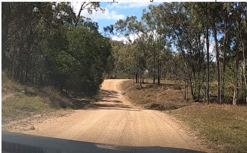
Figure 16 – Unsuitable vertical bend along unnamed road, approximately 2.5km from Mandalee Rd
